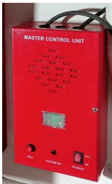
Control Panel with Integrated Hooter – Healthy, Fault, Fire & Discharge Indications.
